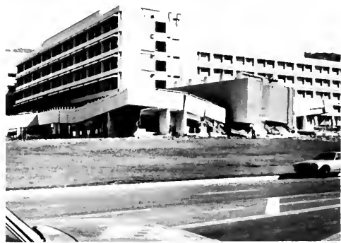
Photo 23. Medical Treatment Building, looking at southwest corner. South stair tower overturned and collapsed on one-story portion; roof at stair tower is center right. Los Angeles City Fire Department photo.
